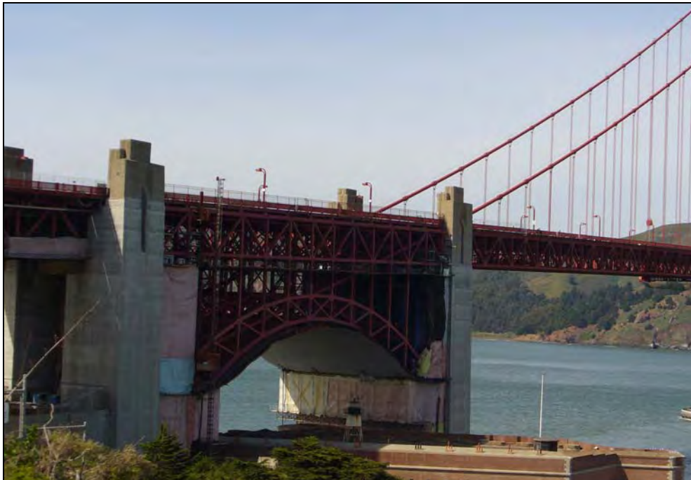
Photograph 7. Seismic retrofit in progress at Fort Point Arch, camera facing northwest, March 2007. [Source: JRP Historical Consulting, LLC]
