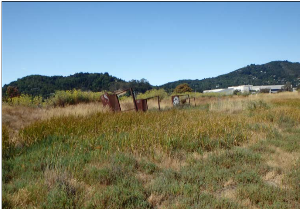
Figure 21. View of the four vertical iron half-cylinder drainage culverts within southwest corner of the ADI, facing west (July 29, 2014).
